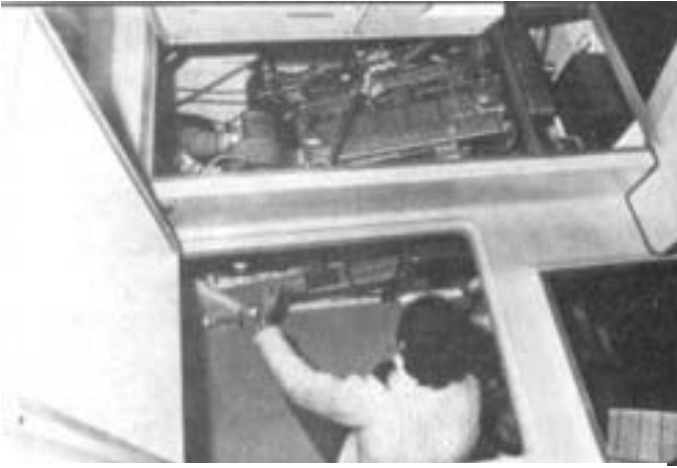
Here the portable panels in the wheelhouse sole have been removed to show the good access to the motors. Even the far side of that port engine can be reached without difficulty.
